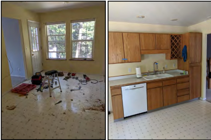
MJ Caswell's kitchen and living room remodel started July 8. "We are all moved over to the guest unit for the kitchen and living room. Lots of work to empty all three rooms so the walls can come down. Walls between living room and dining room are coming out." How exciting!
